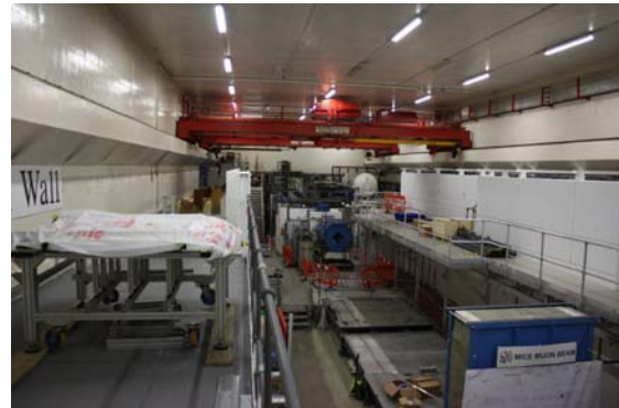
FIGURE 7. View of MICE hall at RAL looking upstream toward the final beam line quadrupole. The muon beam dump appears in the foreground. The cooling channel hardware will be sited in the region in between.
